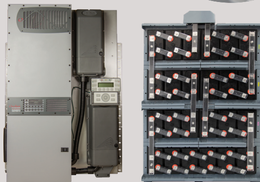
SystemEdge 860XLC-300AFCI FLEXpower Radian & EnergyCell 1000XLC
